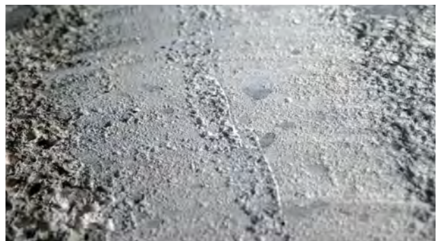
Fig. 6: Crack after impregnation
